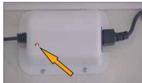
Figure 9B – Charger close-up showing charging indicator light is ORANGE indicating that the lift is connected and is charging.
